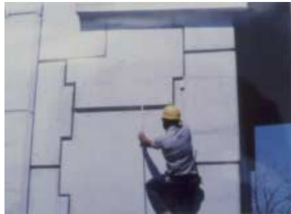
Figure 27, Joints Opening from Settlement
