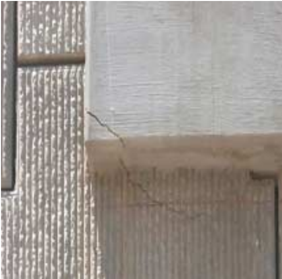
Figure 19, Cracked Panel and Cheek Wall
