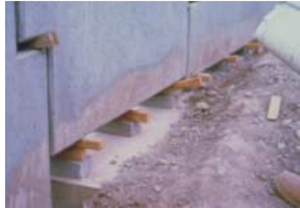
Figure 2, Improper Leveling Pad
