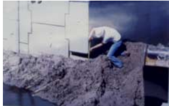
Figure 26, Settlement from Excavation
