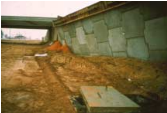
Figure 28, Wall Failure from Exterior Excavation
