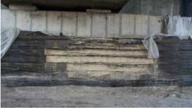
Figure 31, Fire Damaged Reinforcement
