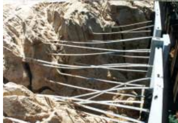
Figure 23, Wash Out From Around Reinforcement
