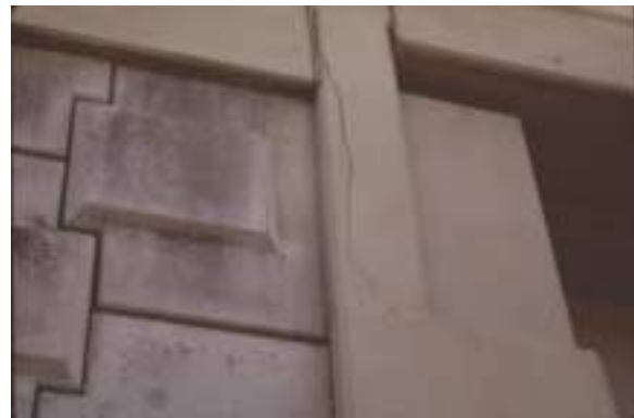
Figure 20, Tension Break in Cheek Wall
