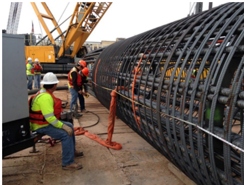
Figure 3.1 Evaluation of steel reinforcement for a drilled shaft (photo by the authors).
