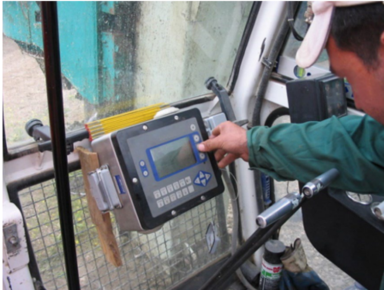
Figure 2-5 Automated Monitoring During CFA Pile Construction (from FHWA GEC 8, Brown, et al, 2007)
