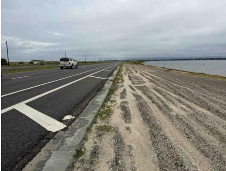
Figure 3-4: Protection of U.S. Highway 98 includes a buried 18-foot deep sheet pile wall and buried gabion mattress.
