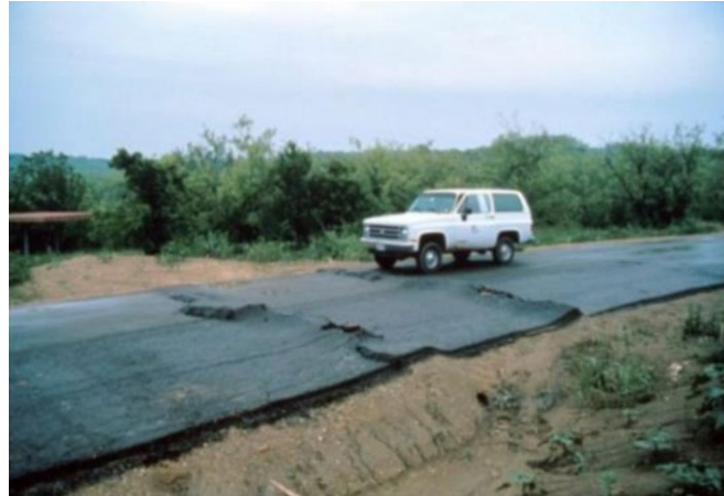
Figure 3-1: Effects of expansive soils on pavements.
