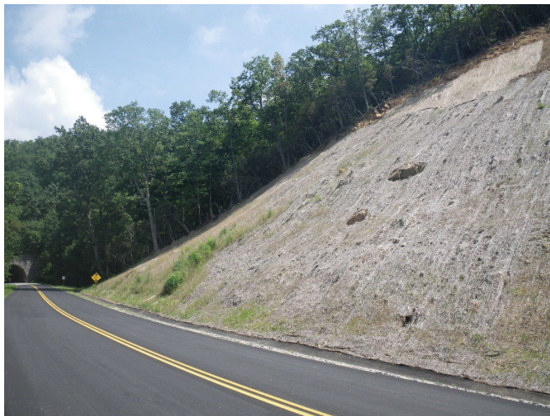
Figure 8-1: Example of slope stabilization mitigation measures. Anchors and slope face stabilization fabric with topsoil and seeds. Blue Ridge Parkway, Henderson County, NC.
