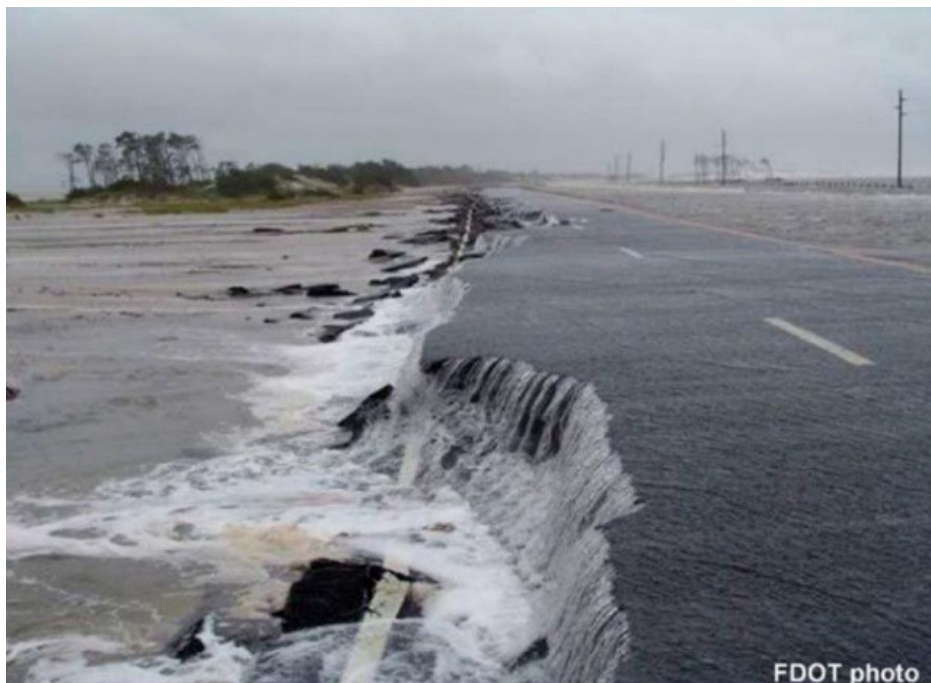
Figure 3-3: Damage to U.S. Highway 98 in 2005 due to a tropical storm (Okaloosa County, Florida).
