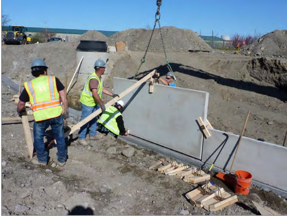
Figure 25: Erection of the first row of facing panels on the prepared leveling pad
