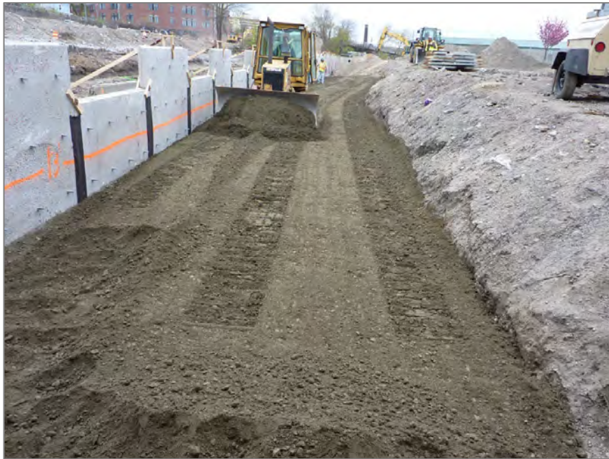
Figure 26: Placement and compaction of reinforced fill on the subgrade to the level of the first layer of reinforcement
